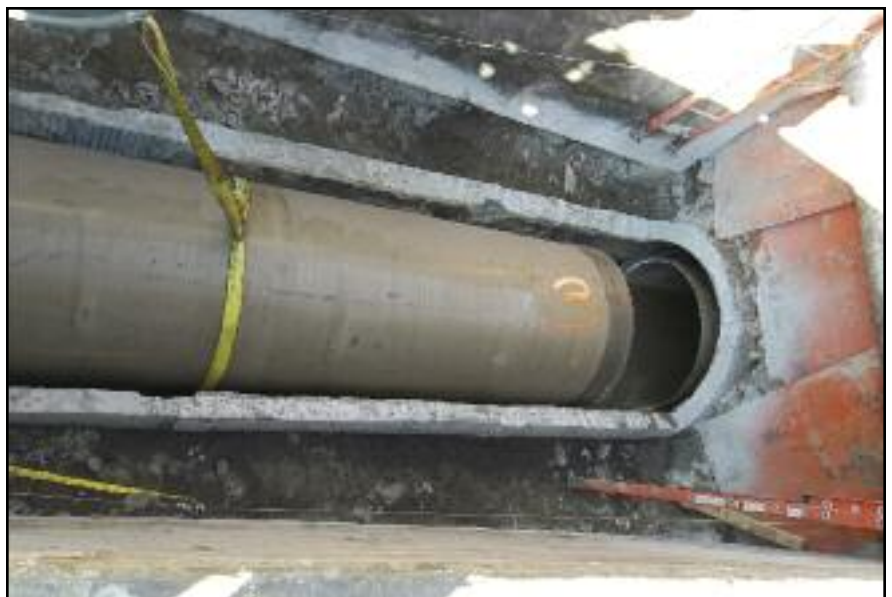
Pipe is lowered into an insertion pit for slip lining in Littleton’s sanitary sewer system.
