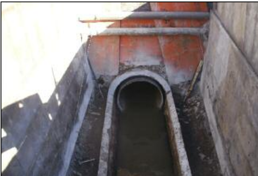
Aging sewer lines need rehabilitation in thriving Littleton.
