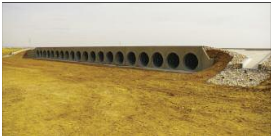
In Artesia, 66-inch corrugated metal pipe was sliplined to rehabilitate old culverts below a highway.
